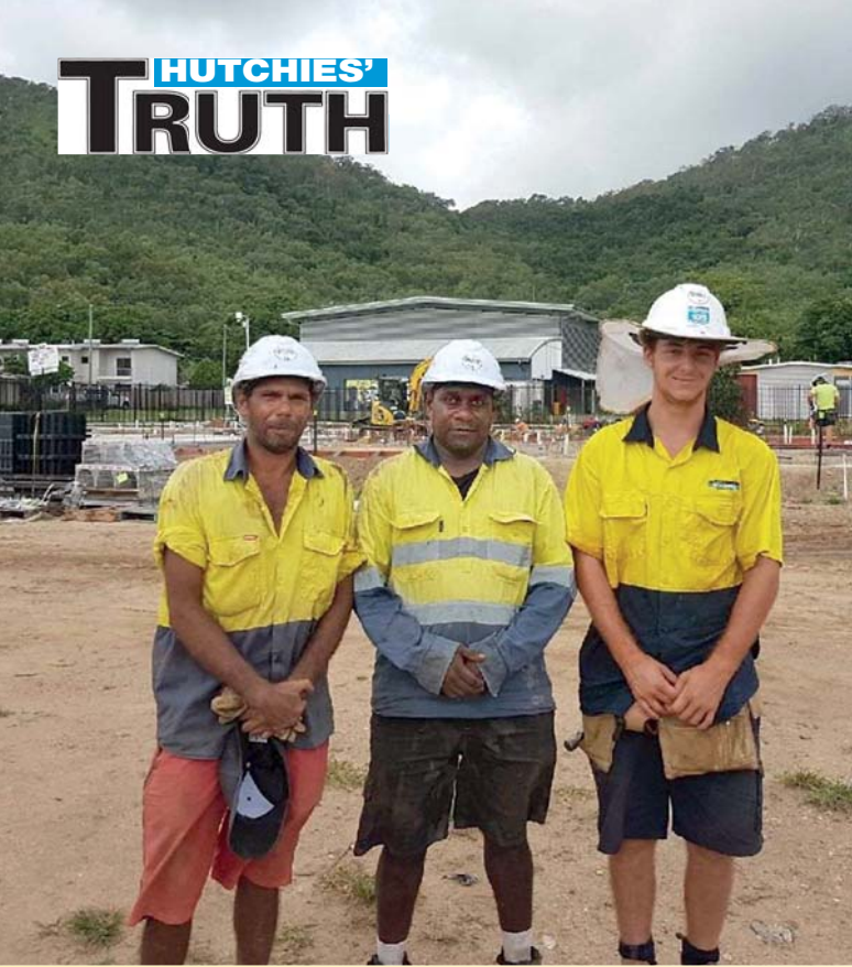
Local team members on the Palm Island project are (from left) Thomas Martin, labourer; Clarence Friday, labourer; and Chance Lively, carpentry apprentice.
