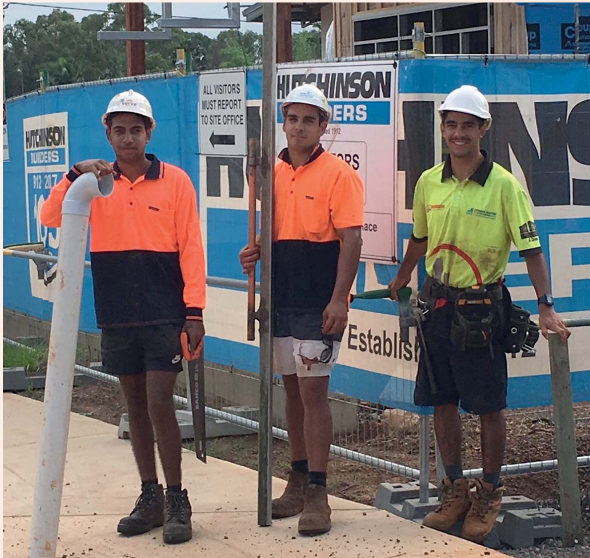
Team members on Hutchies' Howard project (from left) Jamie Warner, plumber; Blayde Foley, concreter; and Scott Carter-Lowe, carpenter.
